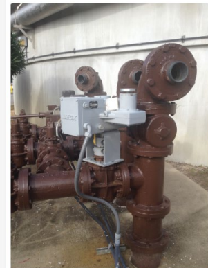
A wastewater treatment plant in Florida uses Beck Actuators on waste activated sludge (WAS) valves in both modulating and open/close service, as well as other areas throughout its treatment process.
